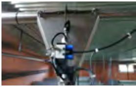
Actuated valve on feeding chains.
